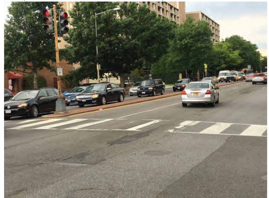
Pavement and markings are in poor condition.
